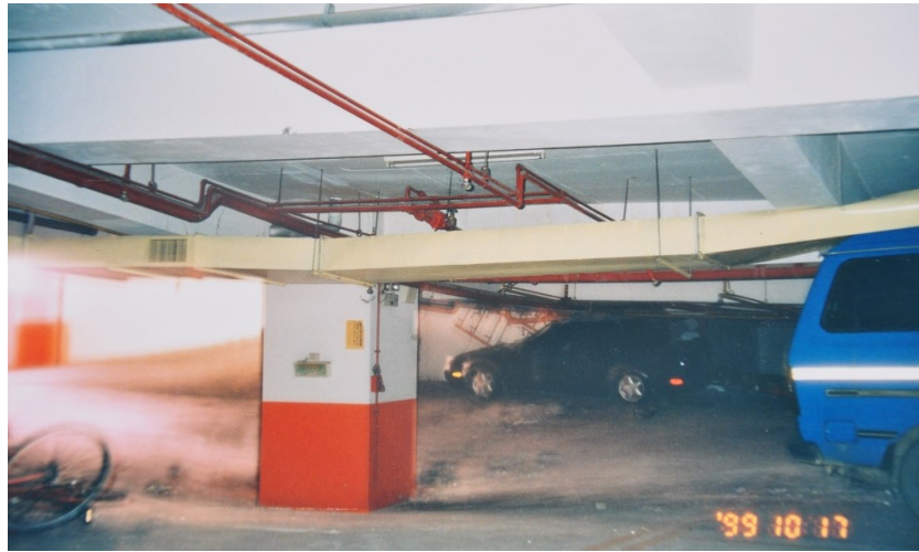
Figure 2. Significant subsidence of the mat foundation of the Haolong Building during the Jiji earthquake (Dongshi, Taichung, Taiwan).
