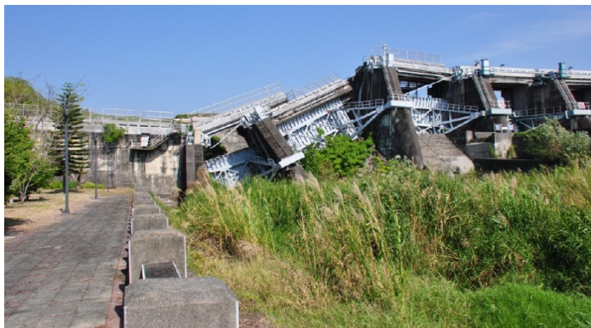
Figure 15. Severe damage to the Shigang Weir resulted from the uplift and tilting effect associated with shear banding.
